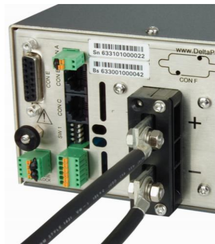
fig 5 - 1 Low resistive cable connection by mounting the cables directly on the DC output strips.
